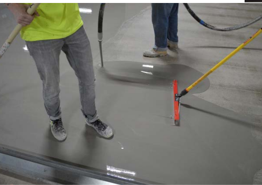
Ardex K 10 — a reactivatable, high-flow, self-leveling underlayment — was used on the floor of this high-technology manufacturing facility in Utica, New York.
