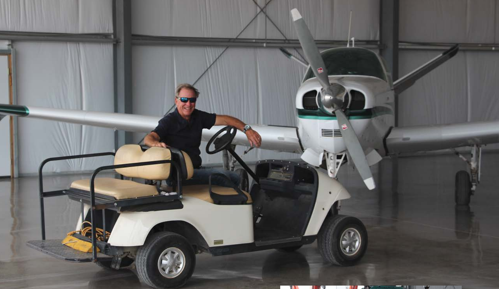
Brad Obbink's company ProFinish employed a power trowel and Superabrasive's Trowel Shine system to polish a concrete floor inside a hangar.
