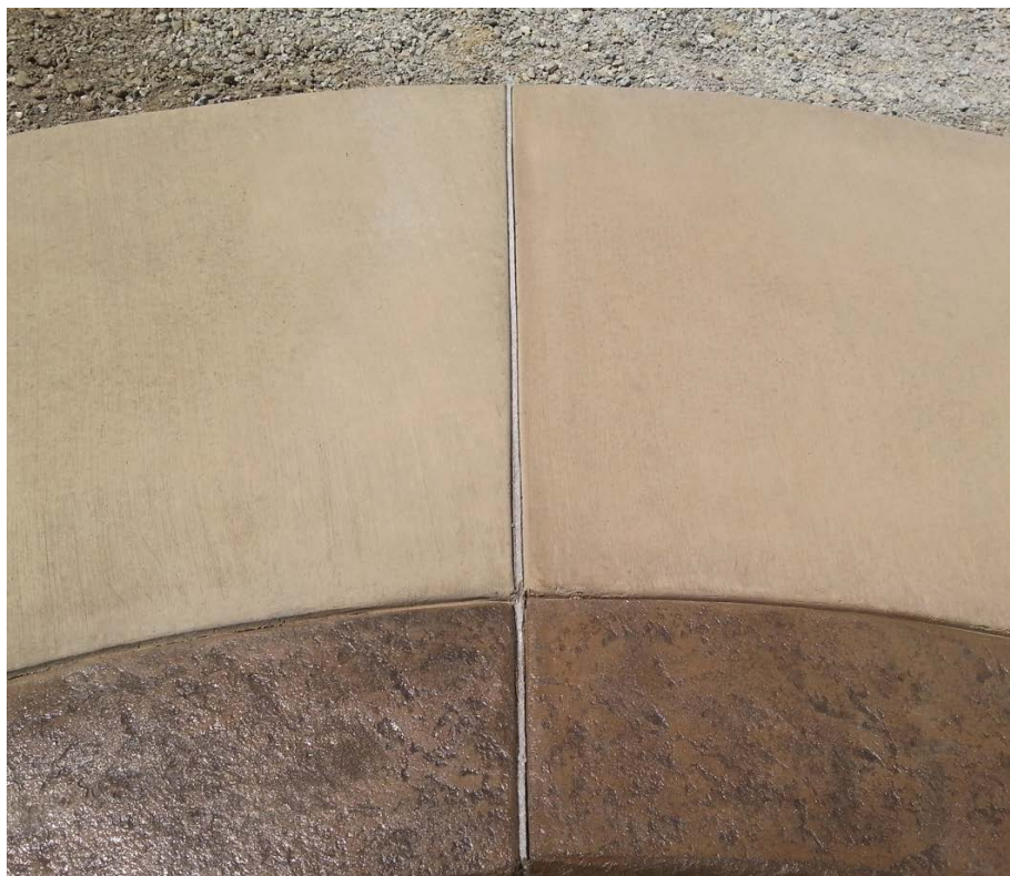
Changing the amount or type of admixture from one pour to the next can lead to color changes in the concrete.
